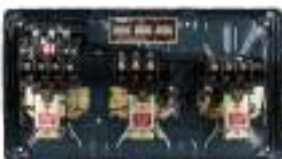
Interior View of MK1 SASD
