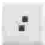
Double RJ 11 Telephone socket
