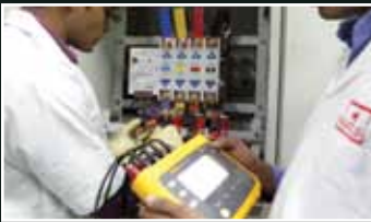
LOAD FLOW & HARMONICS ANALYSIS
