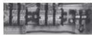
Isolated Terminal blocks for better termination
