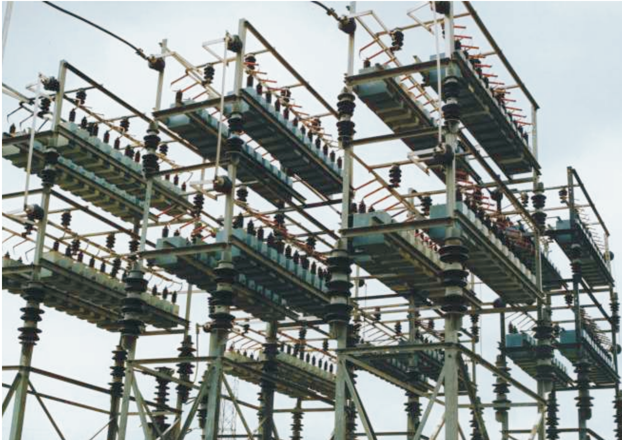
72.5kV, 30MVar, 3 phase, 50 Hz, externally fused, double star connected capacitor bank installation in a 400kV/220kV/66kV utility substation
