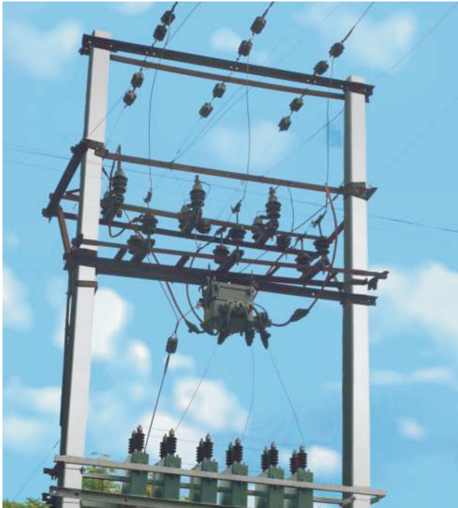
11kV, 600kVAr Automatically switched pole mounted capacitor bank
