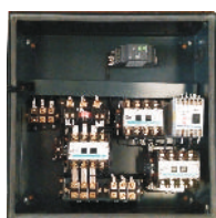
Interior View of MU-G20W FASD
