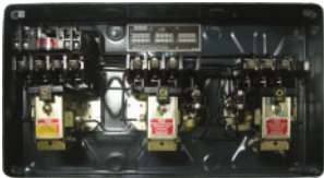
Interior View of MK1 SASD
