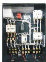
Interior View of MU-G30W FASD
