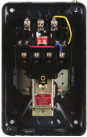
Interior View of MK1 DOL
