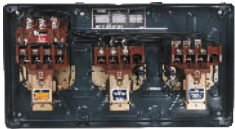
Interior View of MK2 SASD
